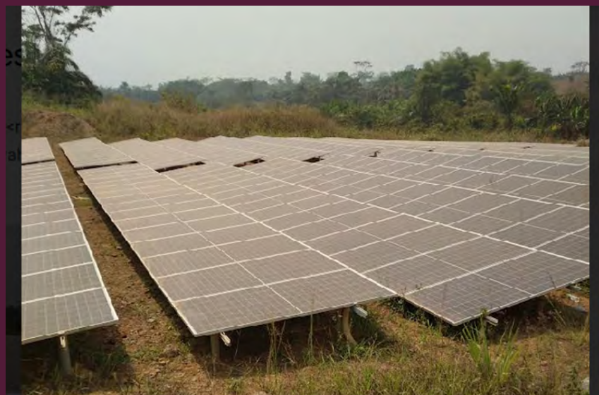
A 100 kWp solar PV system installed at Vester Oil Mills Limited.
